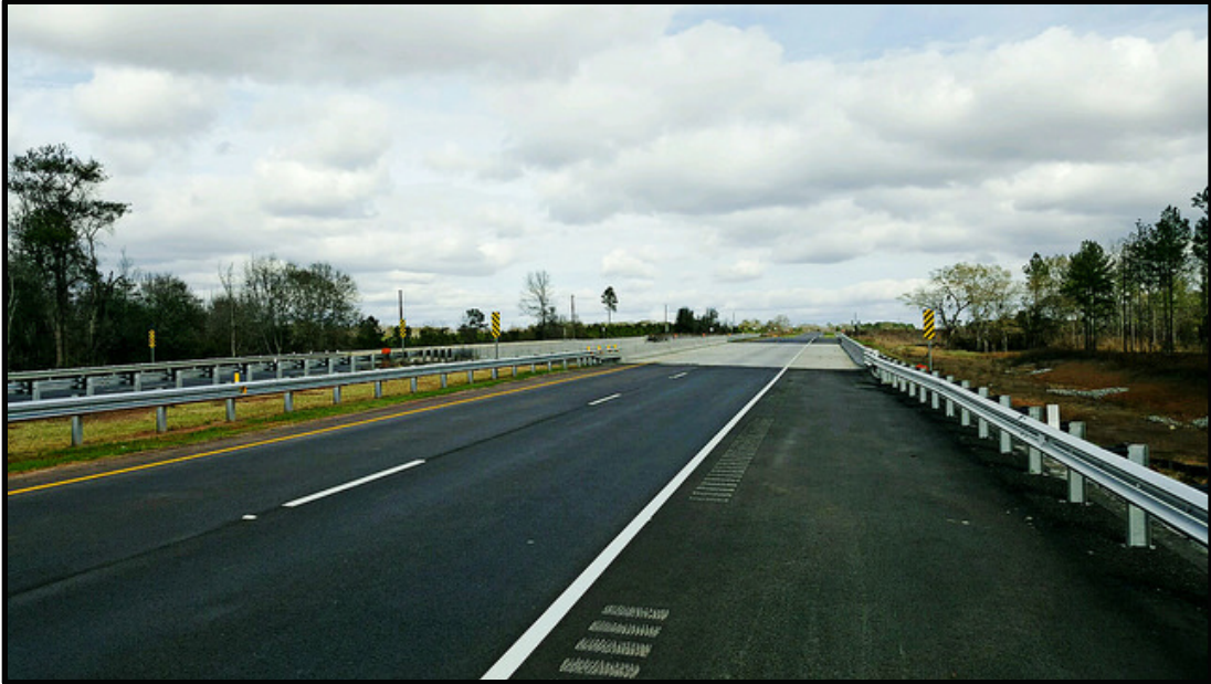
Randolph County, SR1/US27 Widening Project - A 9.13-mile stretch of U.S. Highway 27 south of Cuthbert has been widened to four lanes, creating an alternate north-south corridor to Interstate Highway 75 for motorists. Highway 27 is now four-laned from Indiana to Florida. (Photo: GDOT)
